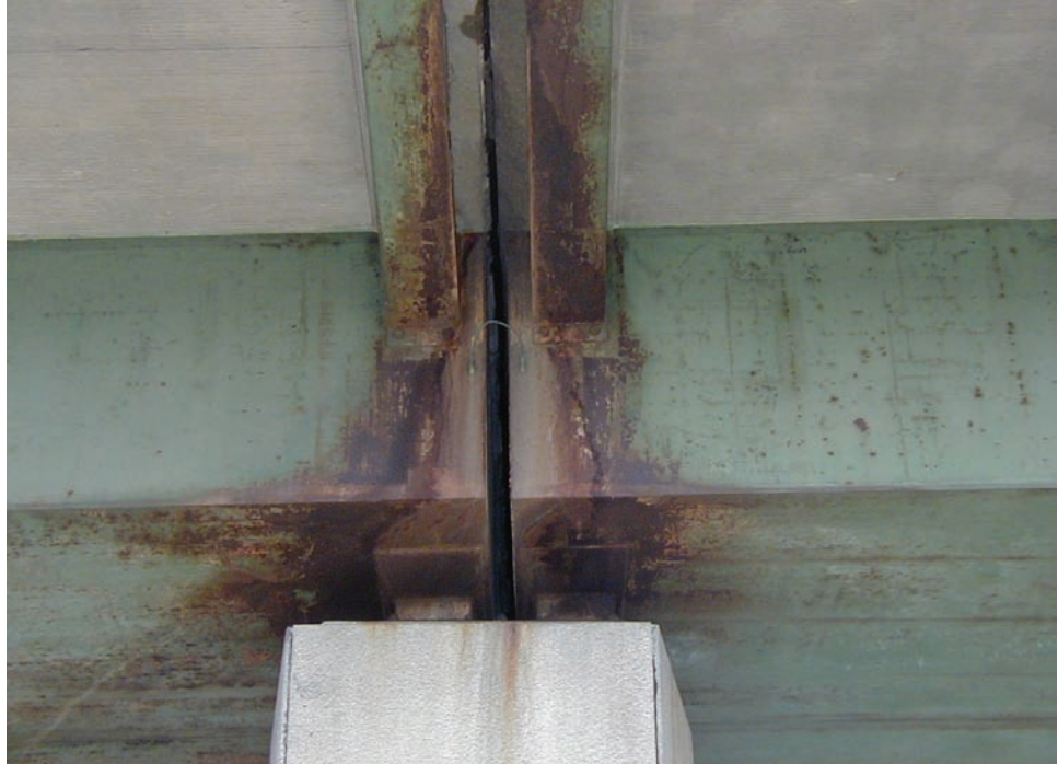
Figure 2.3.19 Water and Salt Runoff Under Expansion Dam Deck Opening
