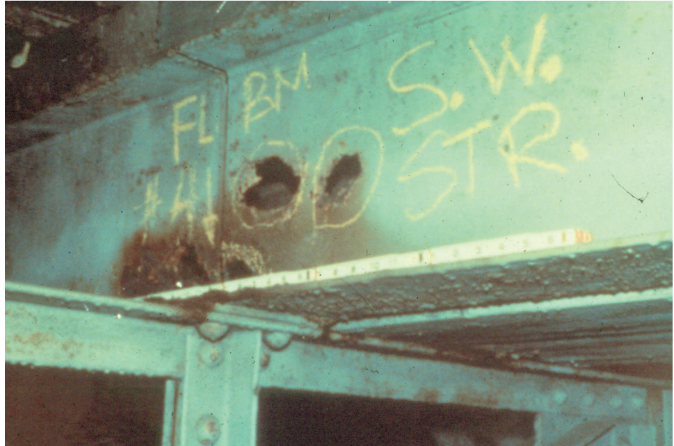
Figure 2.3.6 Steel Corrosion and Complete Section Loss on a Stringer Web
