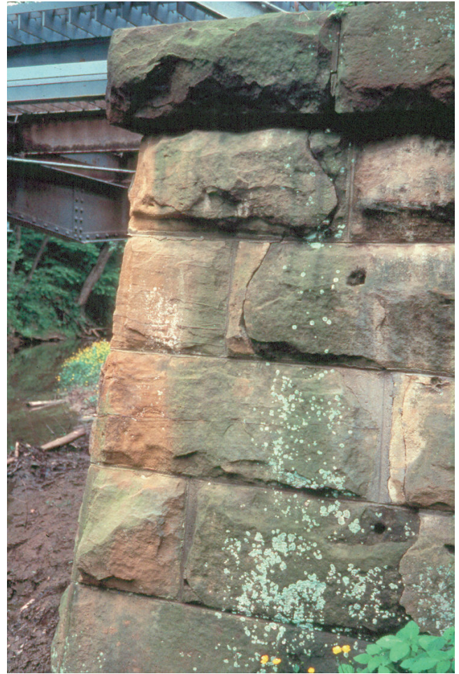
Figure 2.4.2 Splitting in Stone Masonry
