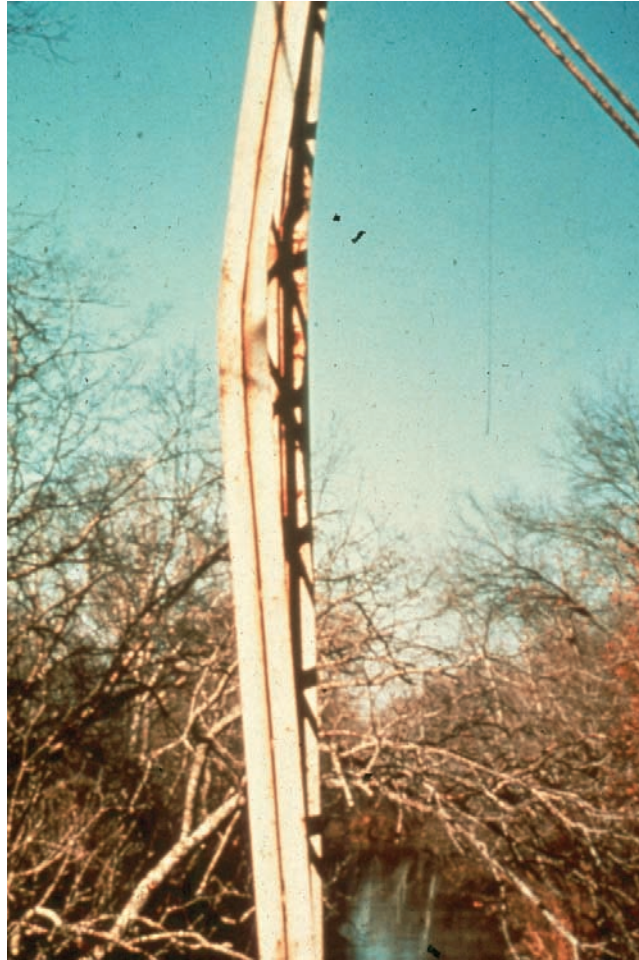
Figure 2.3.9 Collision Damage on a Steel Bridge
