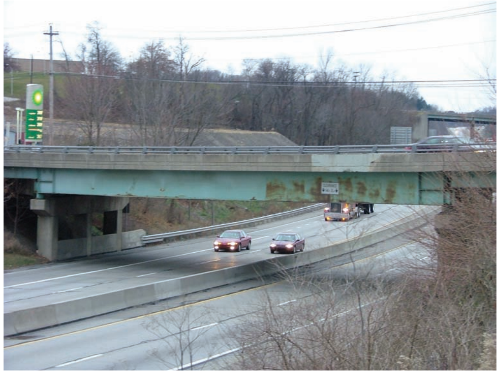
Figure 2.3.21 Roadway Spray Zone Damage
