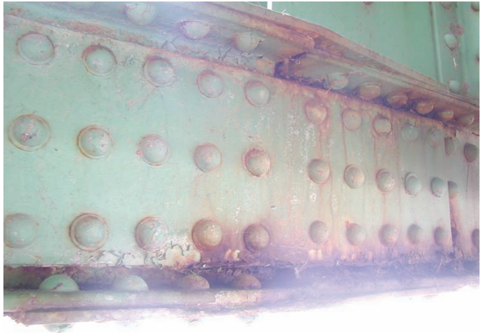
Figure 2.3.20 Corroding Rivet Head
