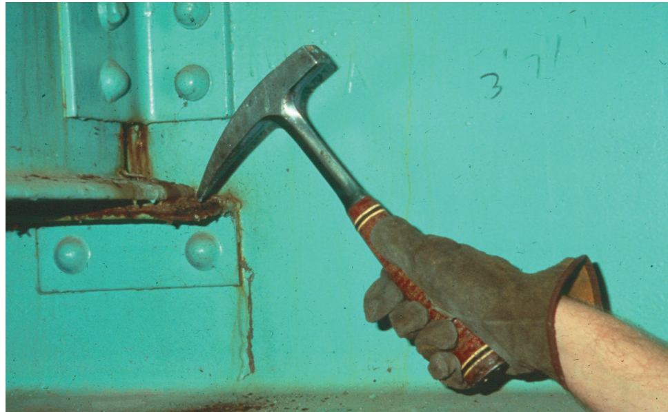
Figure 2.3.16 Corrosion of Steel
