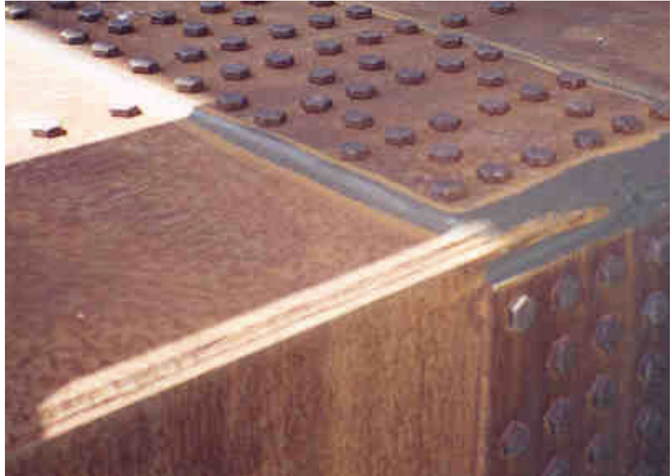
Figure 2.3.24 Light Brown – Early Stage of Exposure
