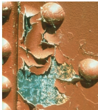
Figure 2.3.14 Paint Peeling from Steel Bridge Members
