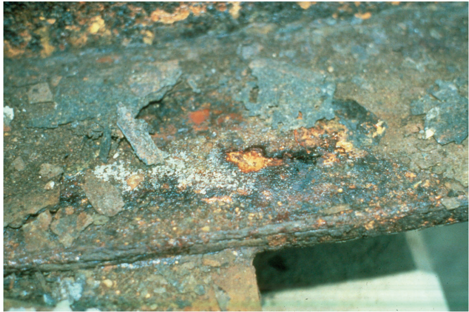
Figure 2.3.22 Color of Oxide Film is Critical in the Inspection of Weathering Steel; Dark Black Color in an Indication of Non-protective Oxide
